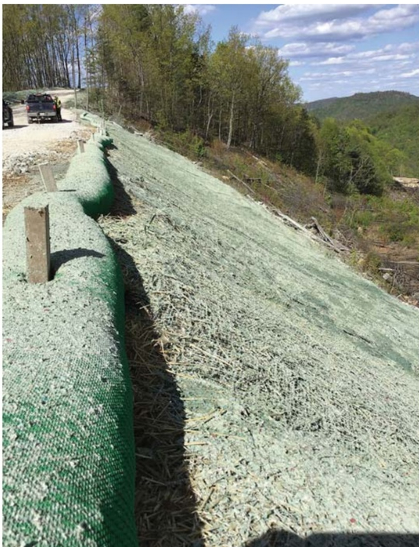
Environmental managers captured this picture with the mapping app. The image depicts a roll that prevents erosion of grass seed and sediment along a mountain road traversing the transmission line project.
